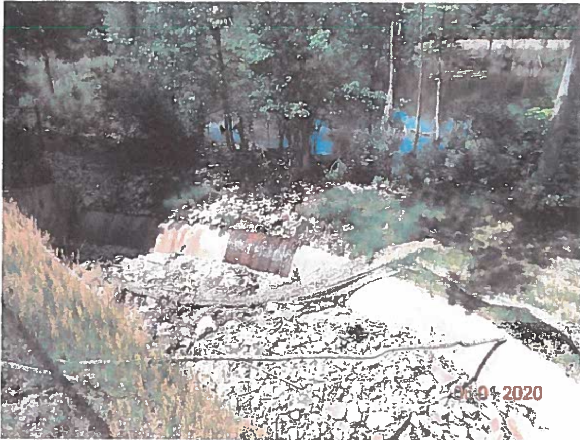
Area above the concrete weir at the inlet end of the triple culverts.
