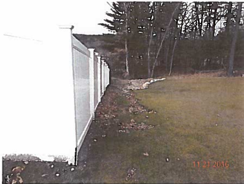
Photo 4: Signs of erosion on Lot 58 (The fence located at the rear of Lot 56).
