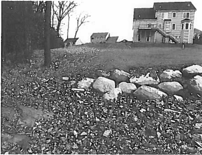
Photo 5: Looking up-gradient from the Open Space to Lot 58. There are signs of erosion on the left (north) side of the slope and accumulated sediment in the lower left of the photo.
