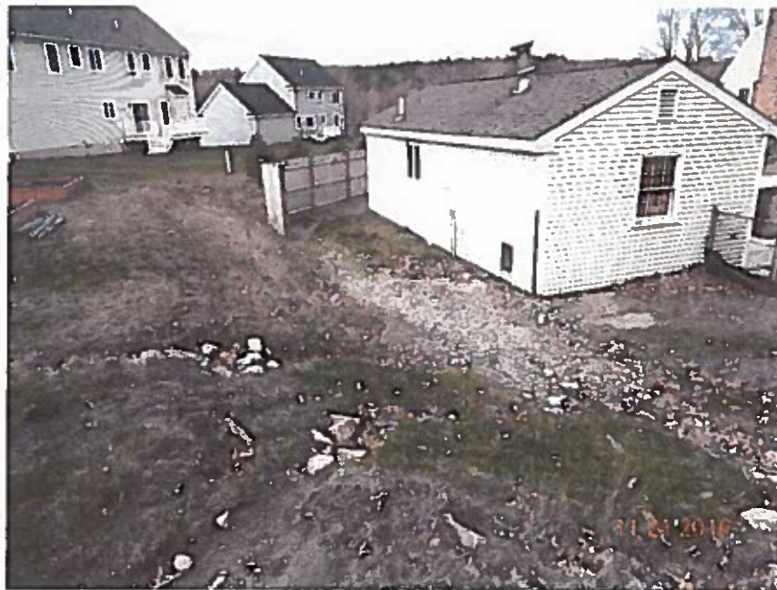
Photo 2: Close-up of sediment deposition on Lot 76. It appears that the deposited sediment is now inhibiting the flow of stormwater around the left (south) side of the building.
