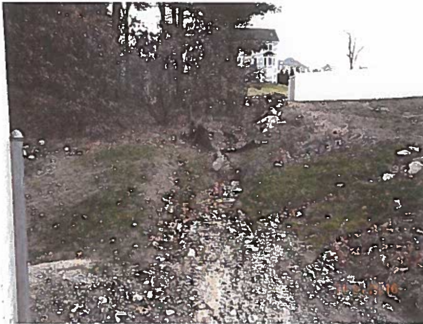
Photo 3: Displaced erosion control barriers and accumulated sediment.
