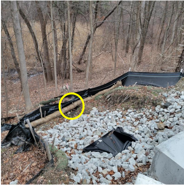
Photo 3: FES-01 installed with a refreshed riprap apron. Note: perimeter controls appear to be undermined in the encircled area.
