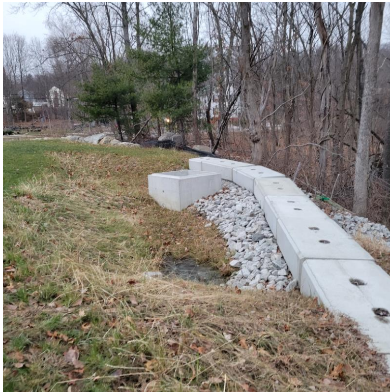
Photo 1: Retaining wall encroaching into basin bottom and the outlet control structure (OCS-101).
